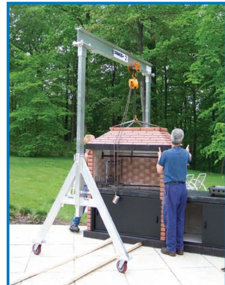
A 2-ton Spanco Aluminum Gantry Crane lifting the top portion of a grill for quick assembly.
