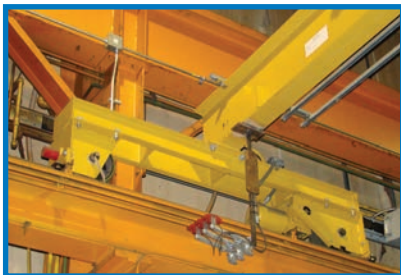
A Top-Running Single Leg Gantry Crane traveling along a ceiling-mounted runway.
